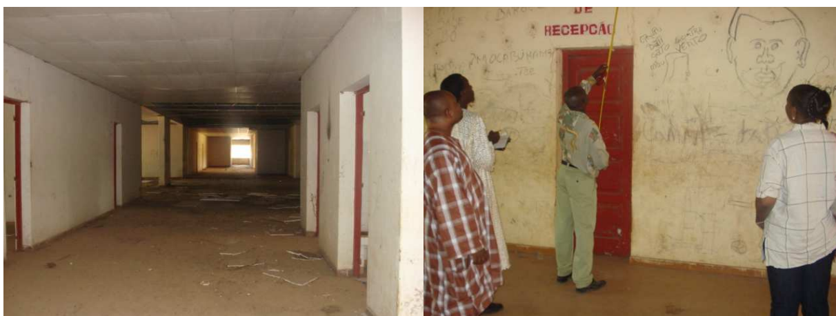
Former Mores Boarding School in na advanced stage of disrepair and
